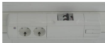
electrical outlet on KB rail.
