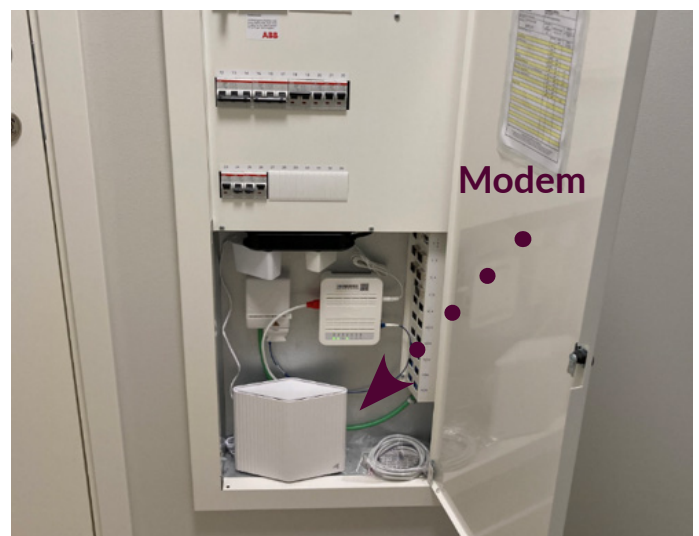
Picture of the fuse box in the hallway
