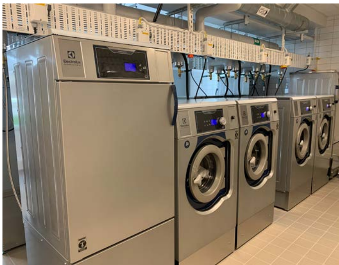
Picture of the laundry room at Fogdevreten 13
