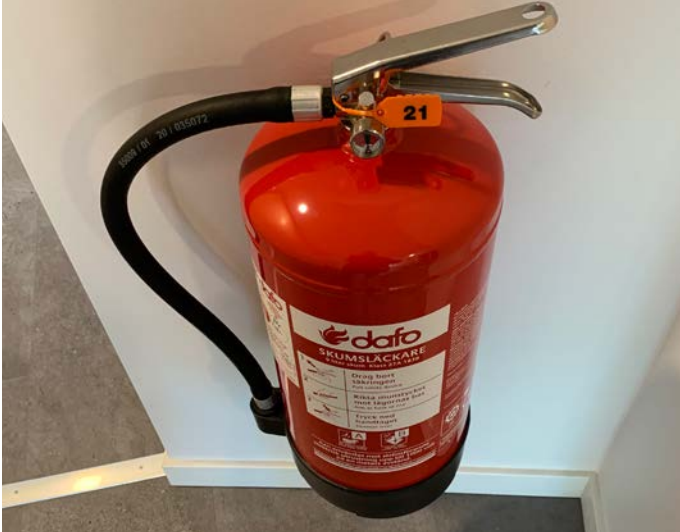
Picture of the fire-extinguisher placed in corridors
