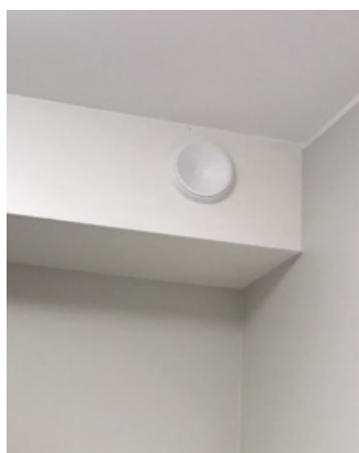
Ventilation in the walk-in-closet
