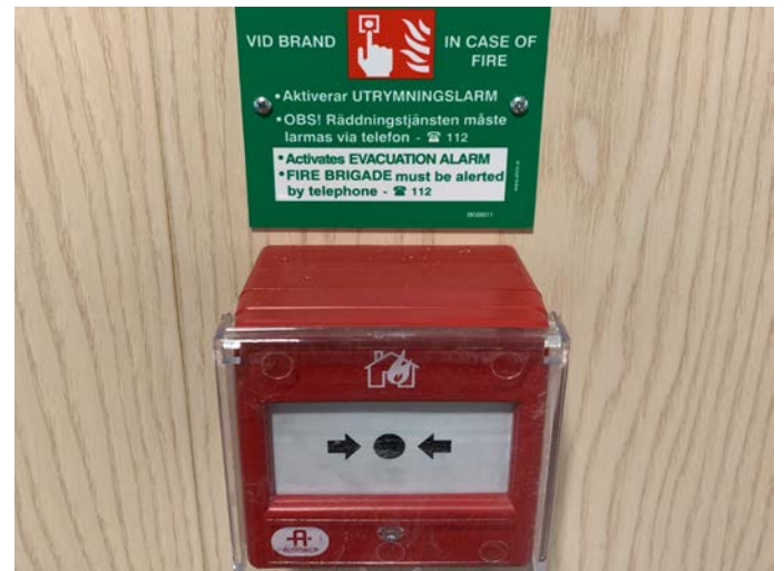
Picture of the alarm switches located in corridors, common areas and entrances.
