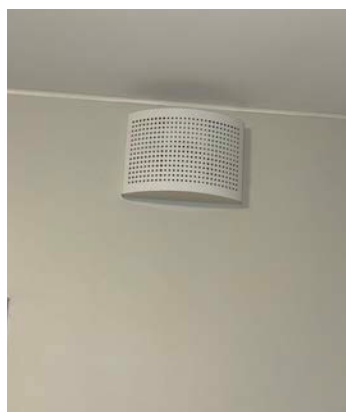
Ventilation in the room
