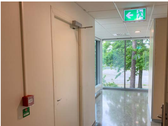
Picture of the door to the evacuation stairs and the emergency exit.
