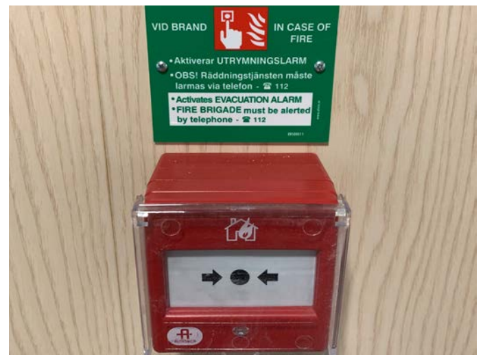
Picture of the alarm switches located in corridors, common areas and entrances.
