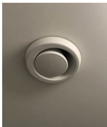
Ventilation in the bathroom
