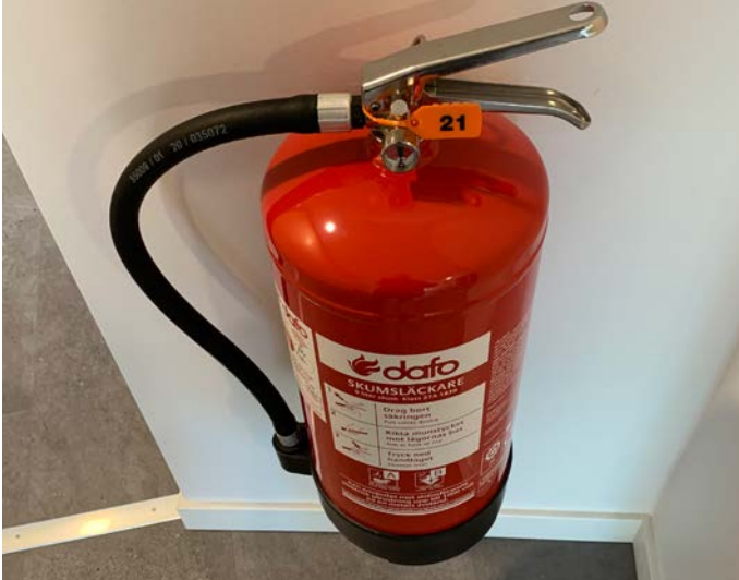
Picture of the fire-extinguisher placed in corridors
