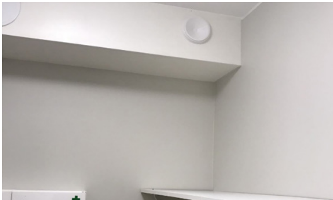
Ventilation in the walk-in-closet
