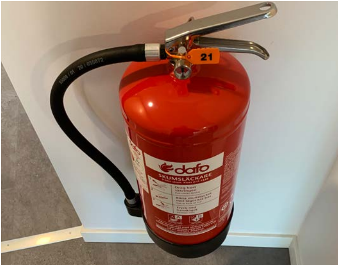
Picture of the fire-extinguisher placed in corridors
