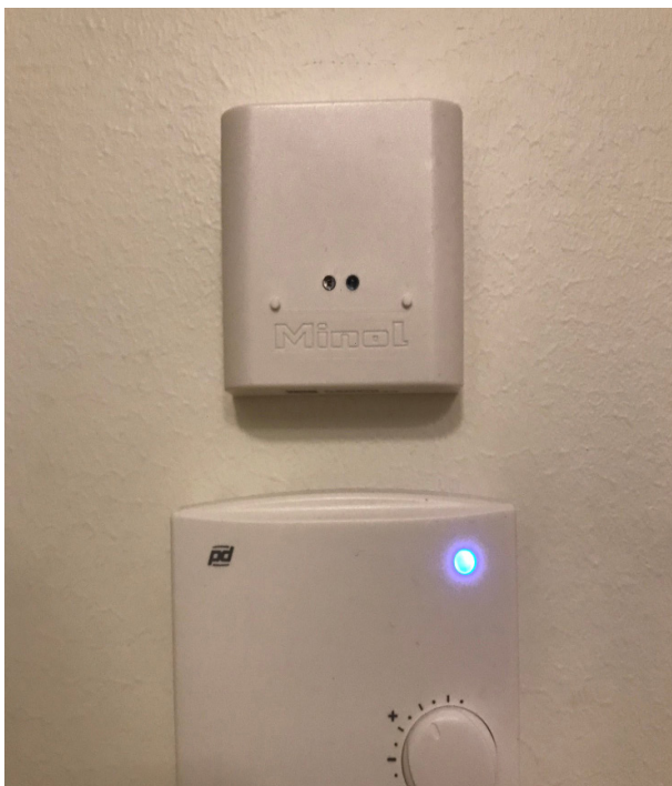
Picture of the thermostat in the apartments
