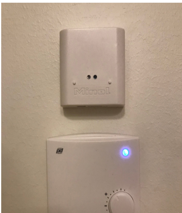
Picture of the thermostat in the apartments
