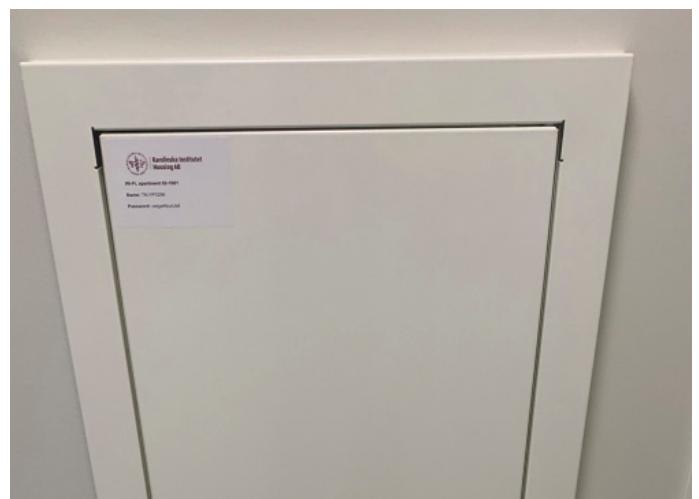
Picture of the WiFi- sticker on the fuse box
