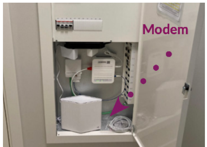
Picture of the fuse box in the hallway
